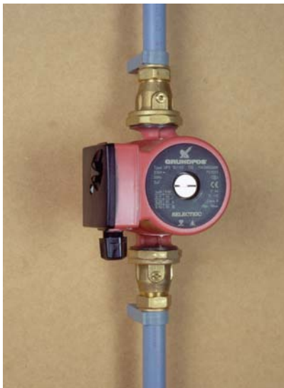
Connection to pump
